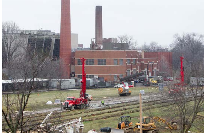
EERE sponsored Ball State University’s campus-wide geothermal system, which is expected to save $2 million annually in operating costs and cut the university’s carbon footprint in half. Here, geothermal boreholes are dug to install the system next to an existing coal-fired power plant. Photo from Ball State
