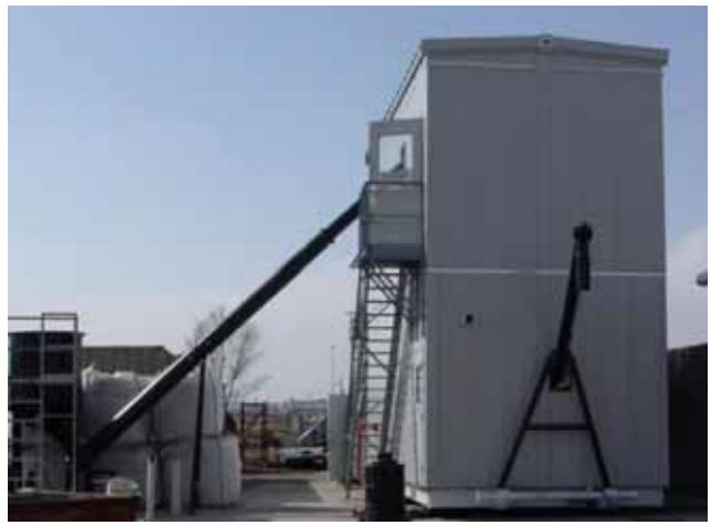
25 ton per day PSRG Gasifier with enclosure, feed auger, and ash shoot
