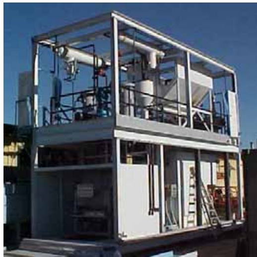
25 ton per day PSRG Gasifier without enclosure, feed auger, and ash shoot
