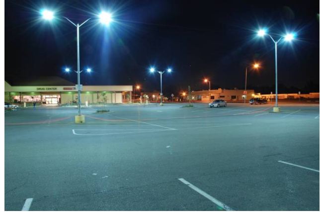
Bi-level parking lot lighting demonstration, Sacramento, California
