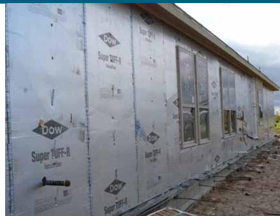
David Weekley Homes covers the building exterior with 1-inch of rigid foam XPS providing a continuous air barrier and thermal break for the building envelope.
